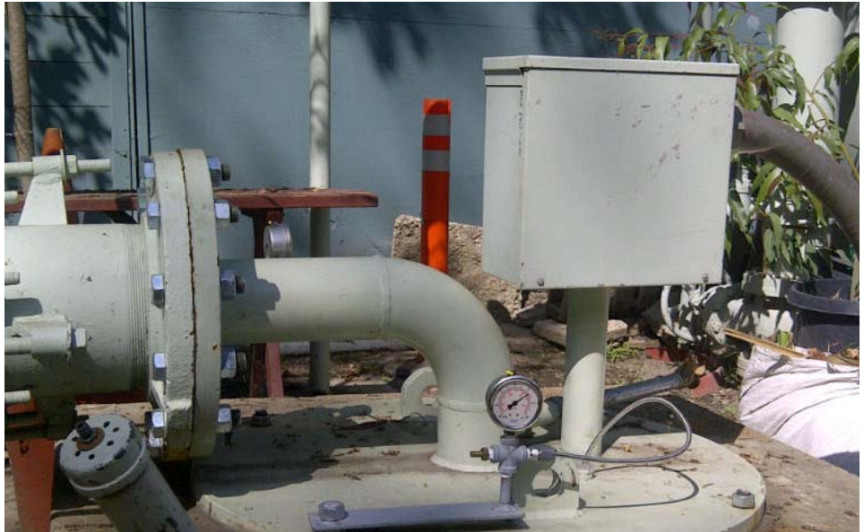
Long way down! A view of our irrigation well head, where our new well pump and motor sits about 300 feet underground.
